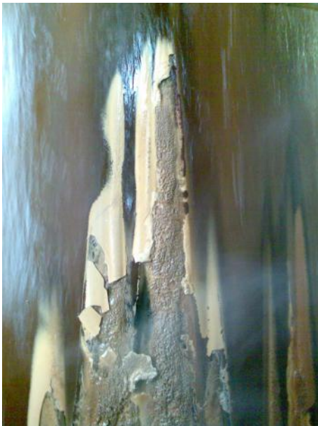
Calcium Carbonate deposits crumbling any brushing or cleaning
