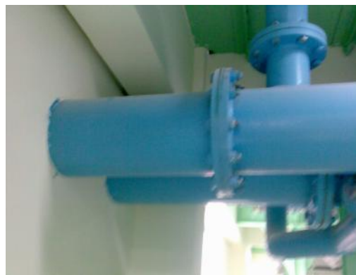
Pipe where MERUS ring is to be installed
