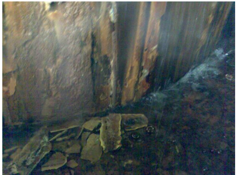
Chunks of calcium carbonate fallen off from the external without furnace wall.
